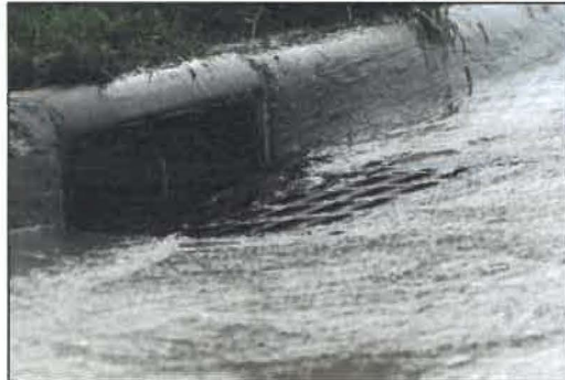
Storm water management
