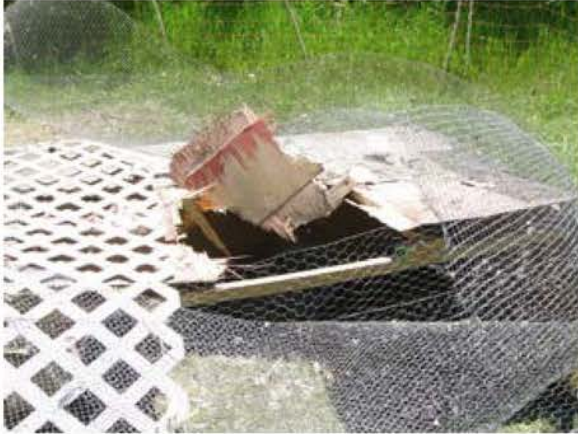
The hole in the roof and the dead chicken the bear hadn't eaten yet.
