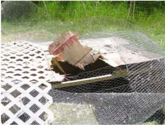
The hole in the roof and the dead chicken the bear hadn't eaten yet.
