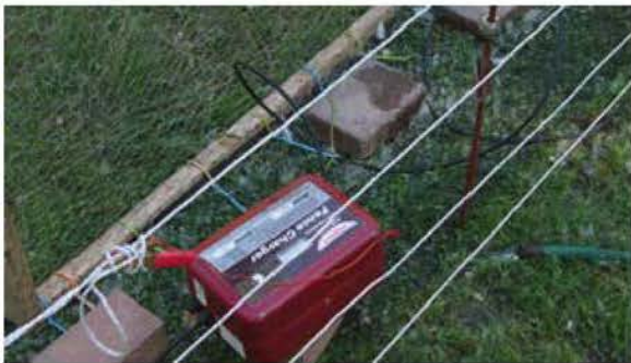
I ran water on the ground rods to make the soil more moist and help with putting a good charge on the fence.
