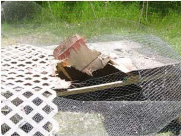
The hole in the roof and the dead chicken the bear hadn't eaten yet.
