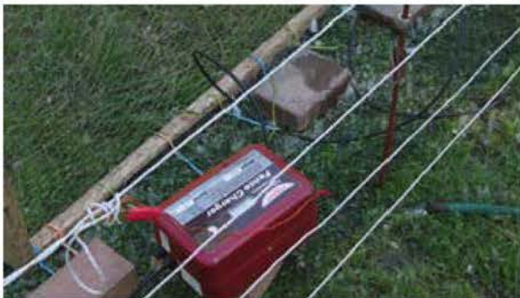
I ran water on the ground rods to make the soil more moist and help with putting a good charge on the fence.
