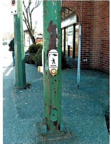
Old Traffic Signal Pole
