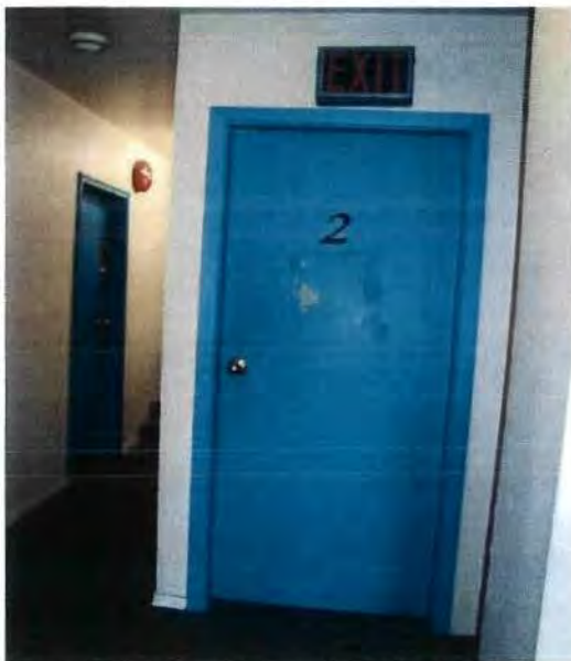
Exit sign above door not illuminated (should be removed in this particular case as the door does not actually lead to an exit)
