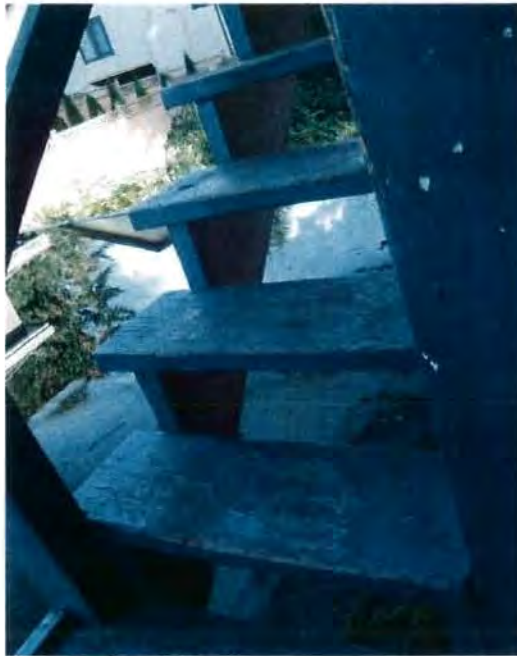
Nonconforming stair rise and runs
