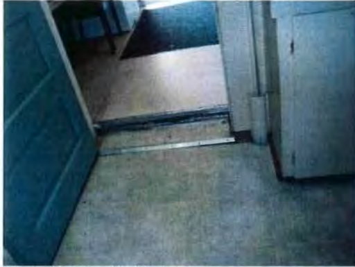
Tripping hazard at door threshold
