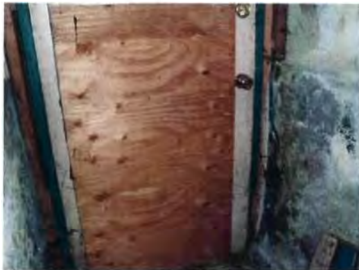
Jammed basement exterior door difficult to open, and has locking device not permitted
