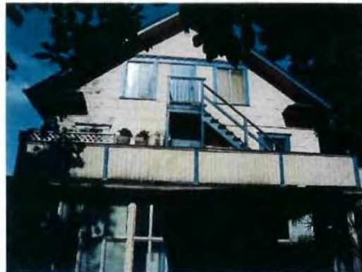
Wired glass in light aluminum frames, openable windows, exposing exterior exit stair
