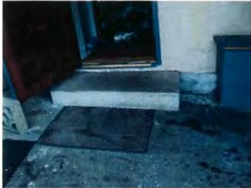
Ground level east suite entrance landing undersized
