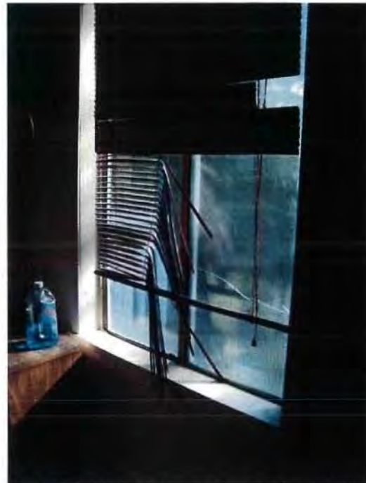
Wired glass in light aluminum frames, glass cracked, openable window
