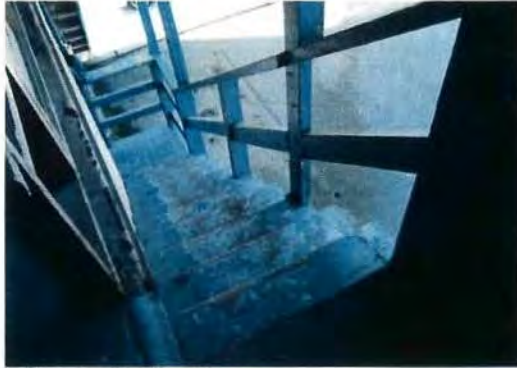
Inadequate exit stair width
