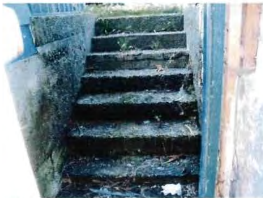
Lack of uniformity in rise and runs
