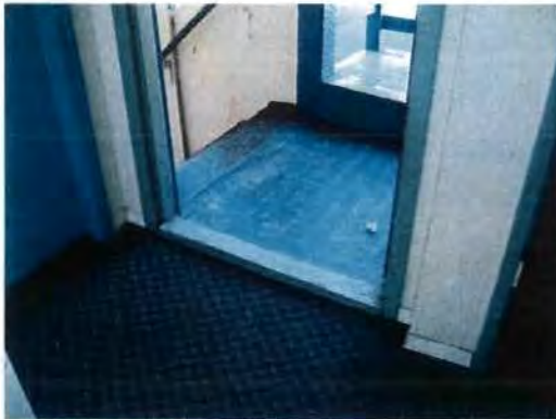
Tripping hazard at door threshold
