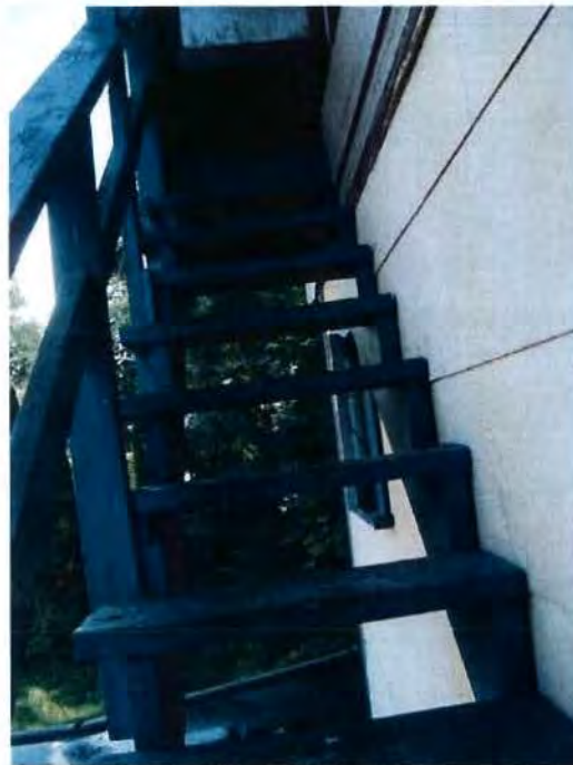
Openings at guards too large, and climbable members present
