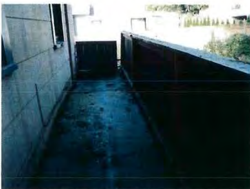
Lateral resistance of guard load needs further assessment
