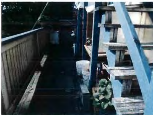
Storage at exterior exit paths
