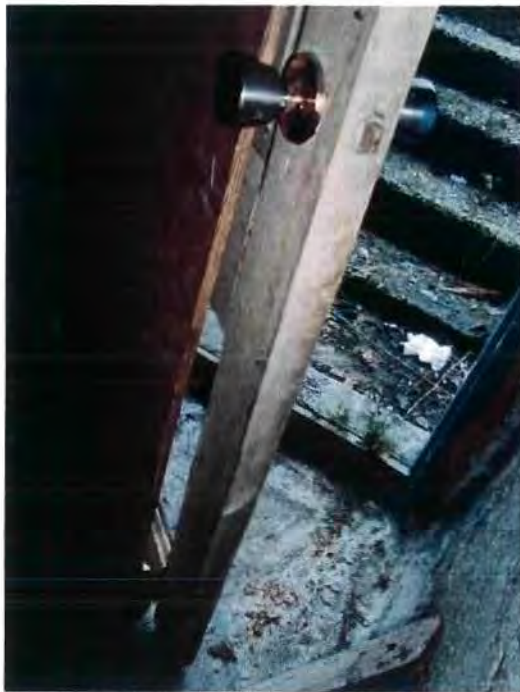
Basement exterior door difficult to open, and needs repair
