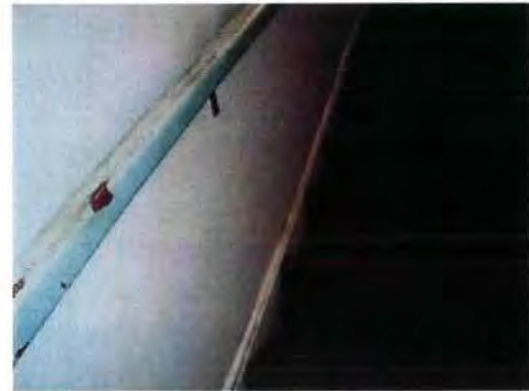
Lack of uniformity in rise and runs
