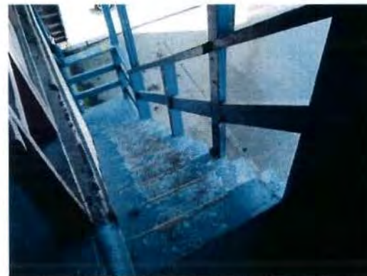
Openings at guards too large, and climbable members present
