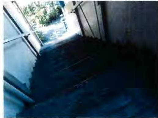
Lack of uniformity in rise and runs
