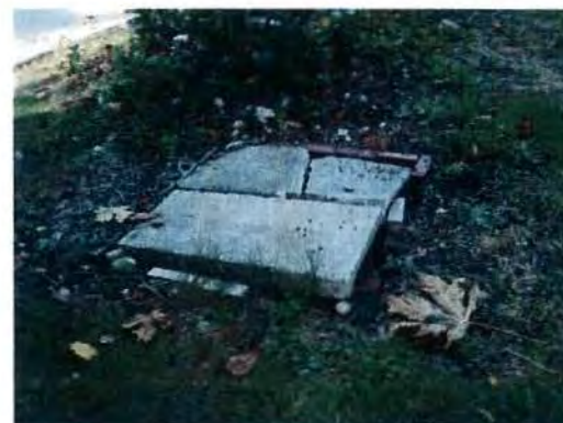
Damaged exterior sump cover presents tripping and fall hazard
