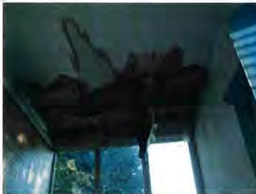
Inadequate repair and maintenance of ceiling fire separation
