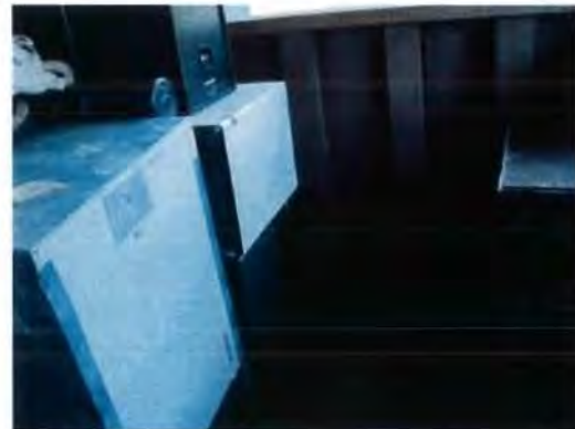
Storage at exterior exit paths
