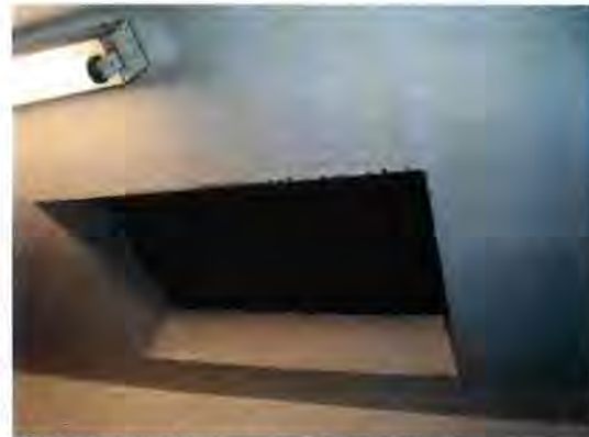
Unrated attic access hatch at fire rated ceiling membrane
