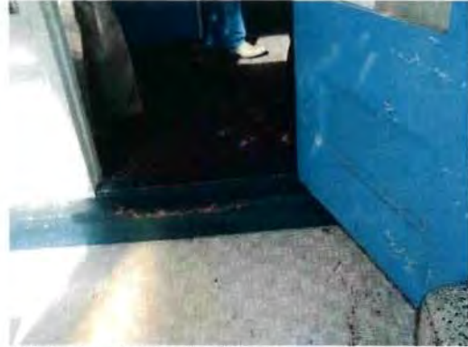
Tripping hazard at door threshold
