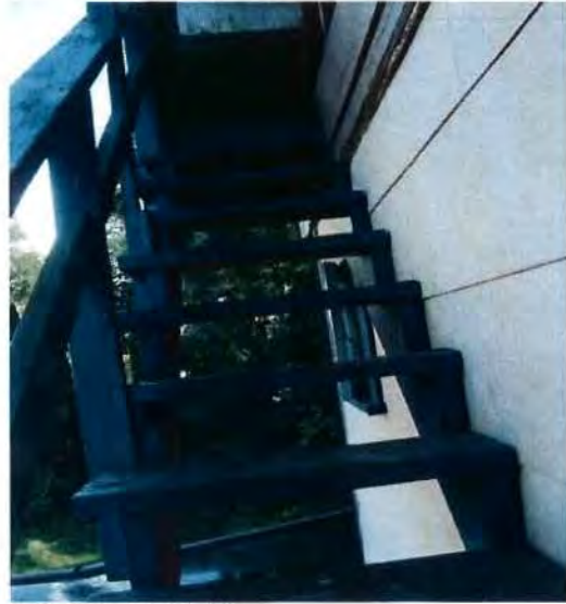
Inadequate exit stair width
