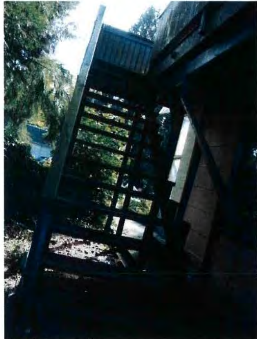
Handrails not graspable
