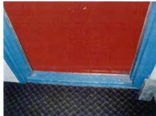
Tripping hazard at door threshold
