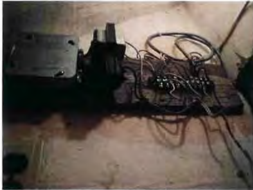
Exposed electrical components at enclosed stair
