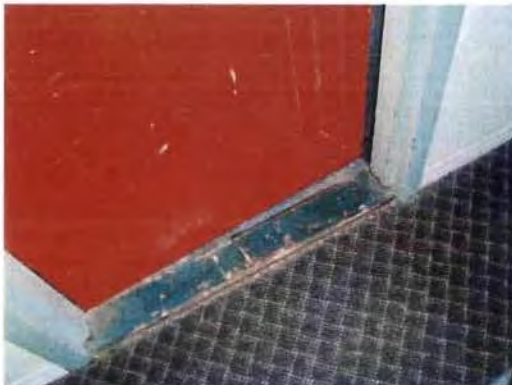
Tripping hazard at door threshold
