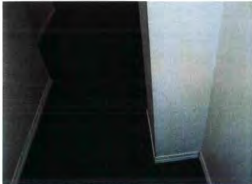
Inadequate public corridor width
