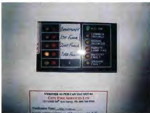
Fire alarm annunciator and control panel
