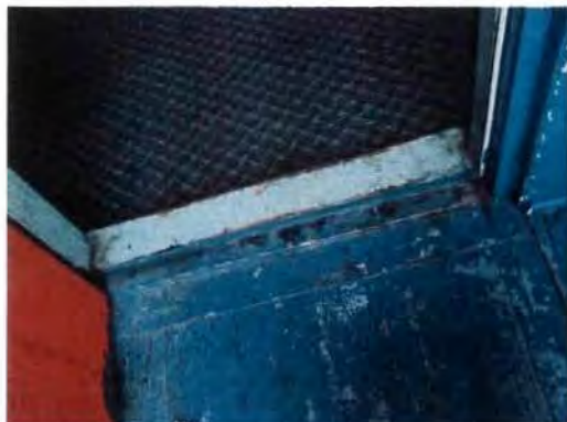
Tripping hazard at door threshold
