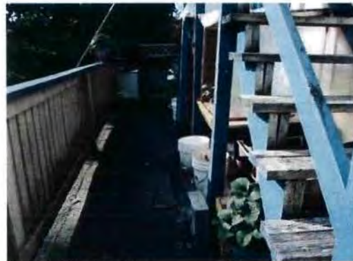
Handrails not graspable
