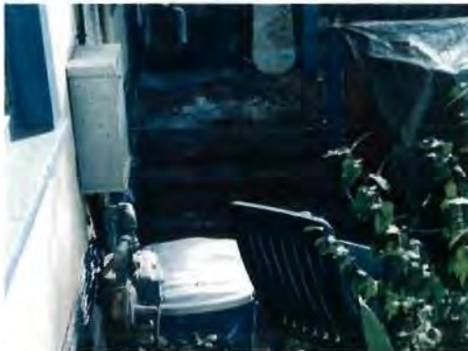
Lack of uniformity in rise and runs
