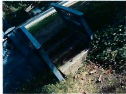
Handrails not graspable
