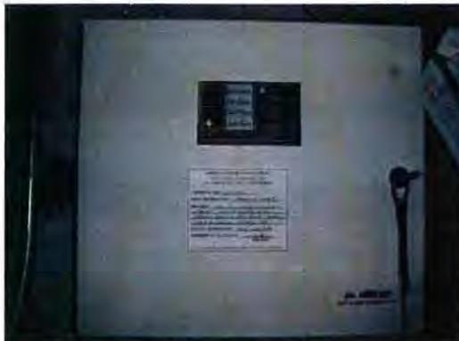
Fire alarm annunciator and control panel
