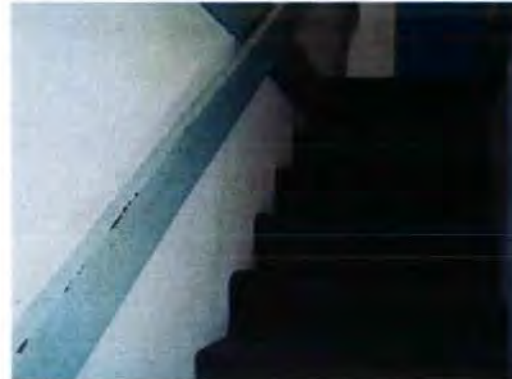
Handrails not graspable
