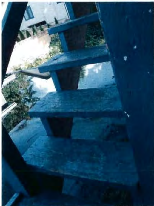
Openings at guards too large
