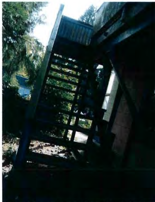
Openings at guards too large, and climbable members present
