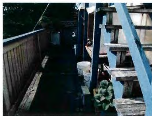
Openings at guards too large
