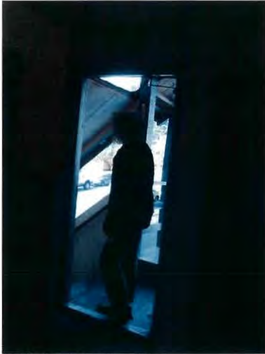
Exit sign above door not illuminated
