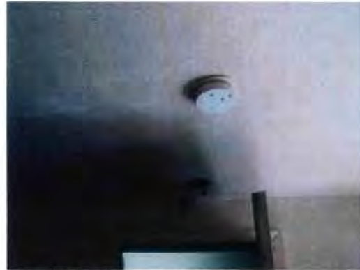
Exposed electrical components at ceiling
