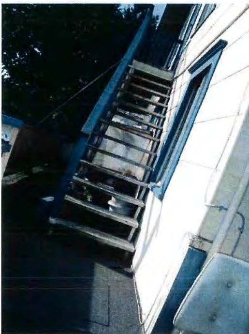
Handrails not graspable
