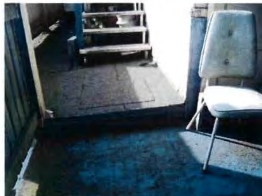
Single step tripping hazard
