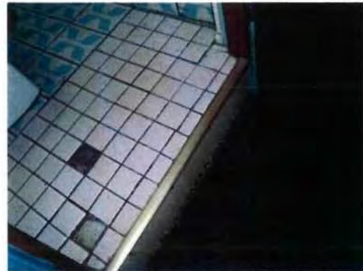
Tripping hazard at door threshold (common area bathroom)
