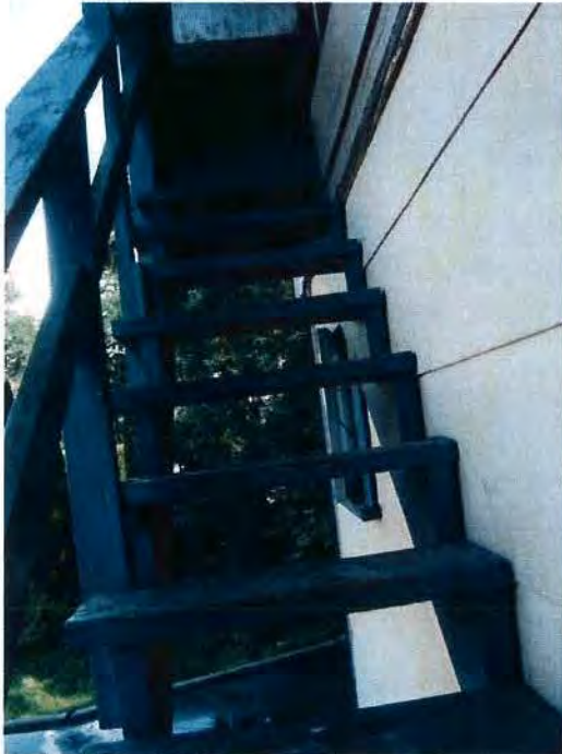
Handrails not graspable
