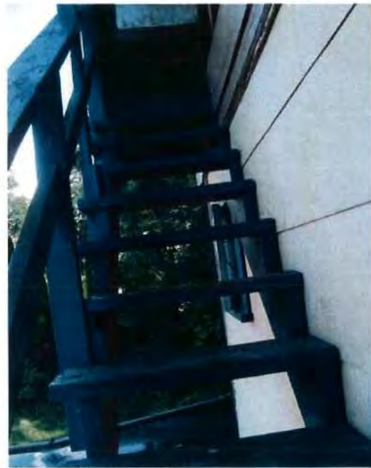
Nonconforming stair rise and runs
