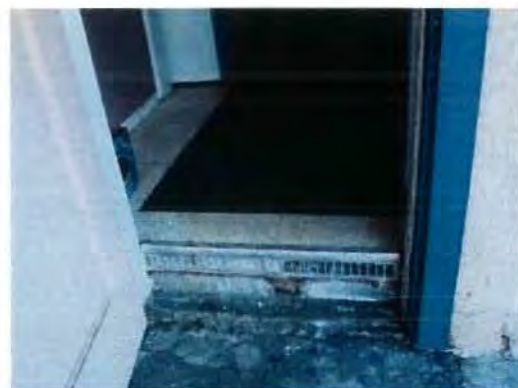
Tripping hazard at door threshold
