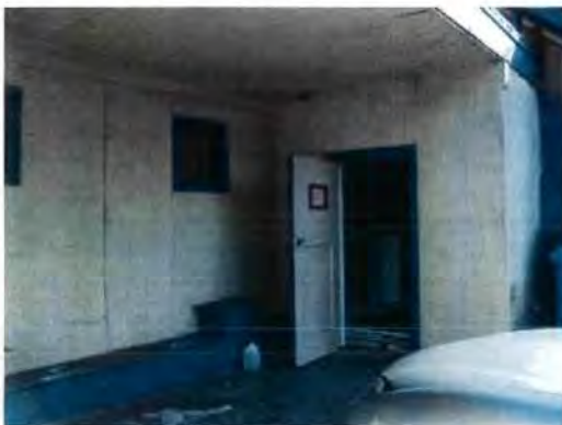
Tripping hazard at door threshold
