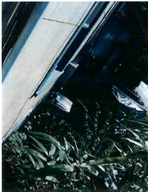
Storage at exterior exit paths
