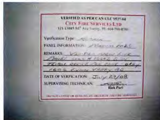
Fire alarm annunciator and control panel
