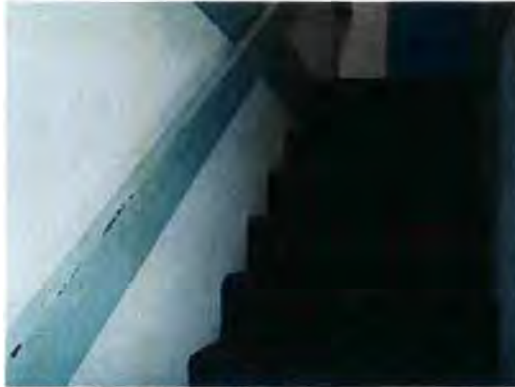
Lack of uniformity in rise and runs
