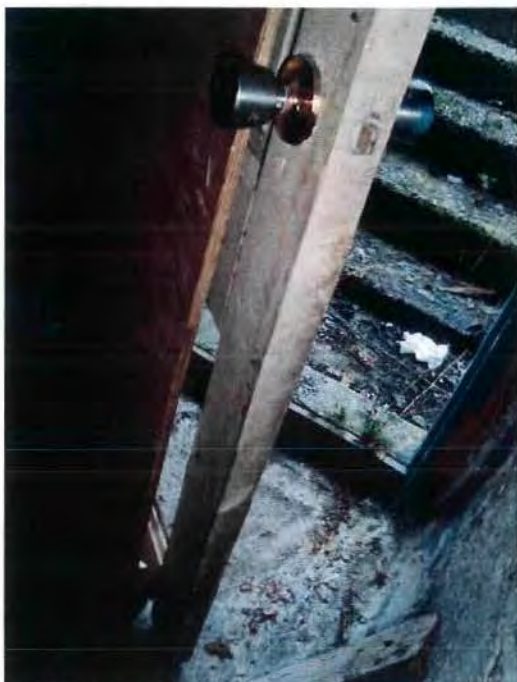
Single step tripping hazard at threshold, basement exterior exit door
