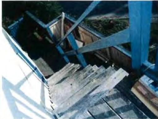
Storage at exterior exit paths
